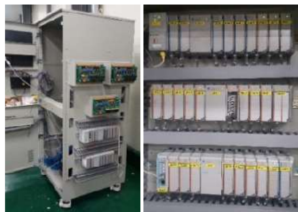
Figure 9: PLC-based PMS functional test simulator: Outer shape with PMS units(Left) and installed PMSIM-V2 PLC system(Right)
