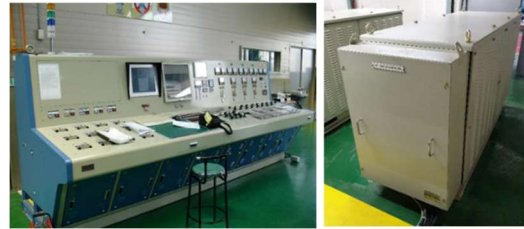
Figure 1: Test console & test generator
