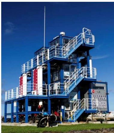
Figure 1: Ocean Thermal Energy Conversion Demonstration Test Facility in Okinawa, Japan
