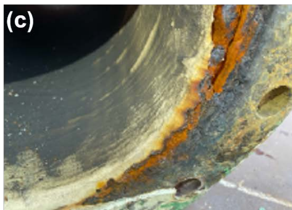
Figure 1: (a) Schematic of overboard pipe, (b) top view of flange surface with the unpainted area, and (c) corroded pipe
