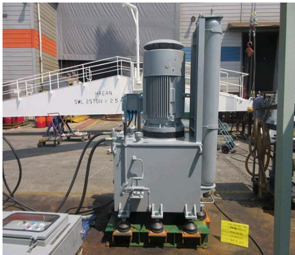
Figure 4: Hydraulic power unit
