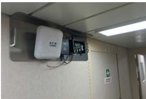
Figure 9: Example of installed RFID reader and UHF module on the ship
