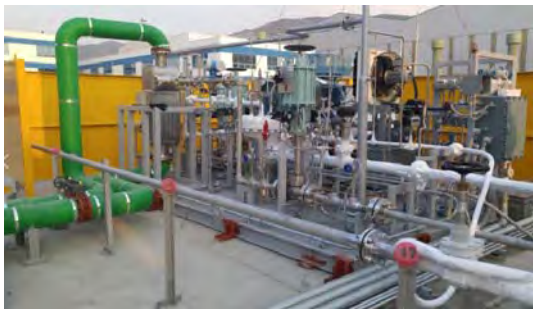
Figure 3: Fuel gas supply system test facility [9]
