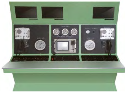
Figure 10: Remote control system
