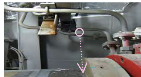
Figure 3: Laser displacement sensor allocation
