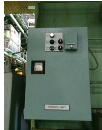
Figure 6: Dosing unit including dosing pump
