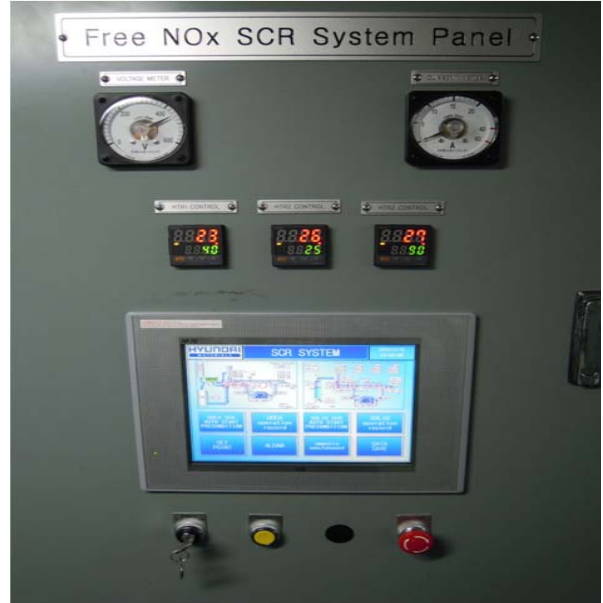
Figure 6: A PLC panel for the SCR system
