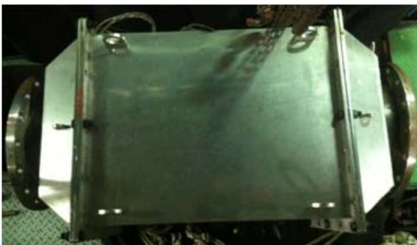
Figure 5: The SCR reactor
