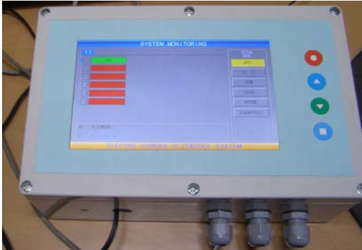
Figure 11: System Monitoring of Master Controller
