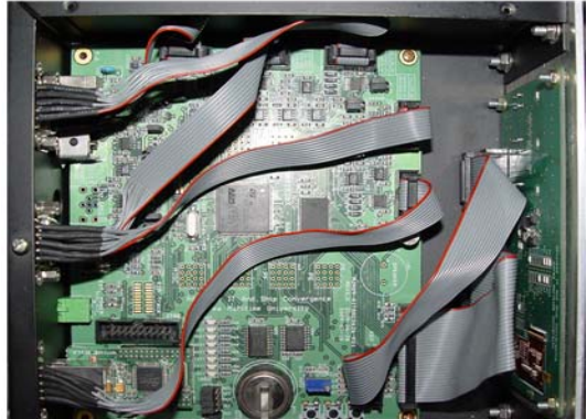
Photo 1: Photograph of engine room monitoring system
