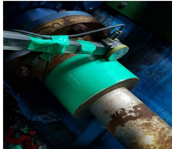
Figure 2: Installation of roller encoder at the propeller shaft
