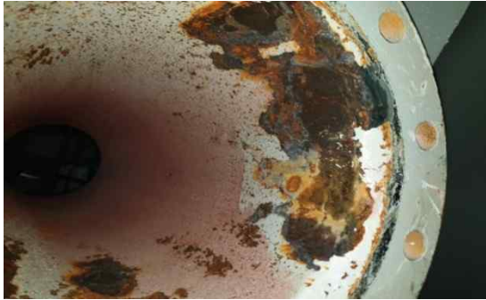
Figure 2: Corrosion around welds in distance piece and bluff body corrosion.
