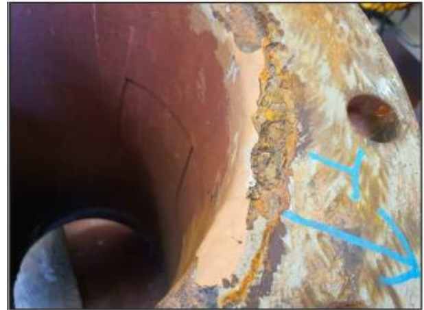
Figure 7: Feature of corroded pipe in the ship
