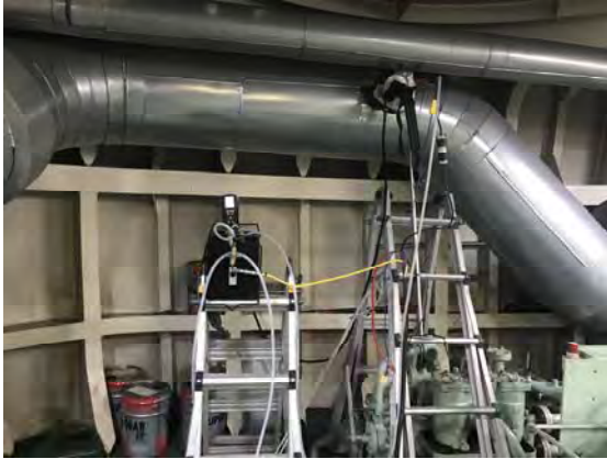
Figure 2: Exhaust emission measurement
