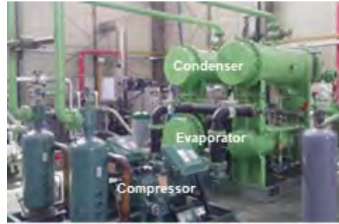
Figure 1: Experimental equipment of the seawater cooling system
