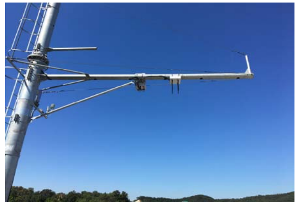
Figure 4: The road side station for WAVE communication
