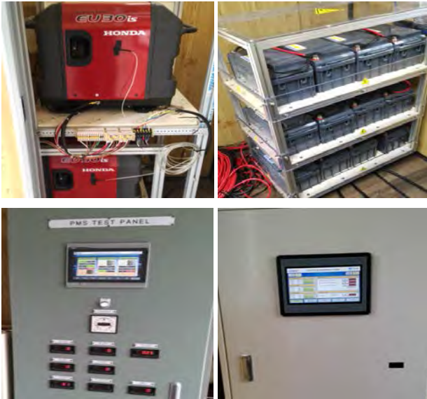
Figure 6: Photograph of generation parts and panels
