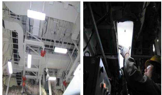
Figure 3: Photograph of the LED luminaires
