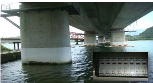
Figure 6: Ti-Mesh anode ICCP system of bridge piles
