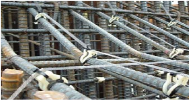
Figure 5: Tied MMO/Ti-Ribbon anode up the rebar
