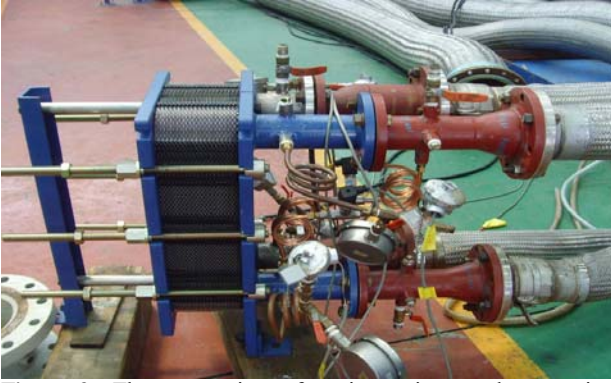
Figure 3: The connection of various pipes and measuring devices
