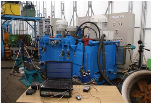
Figure 3: Vertically installed HPU without shield chamber
